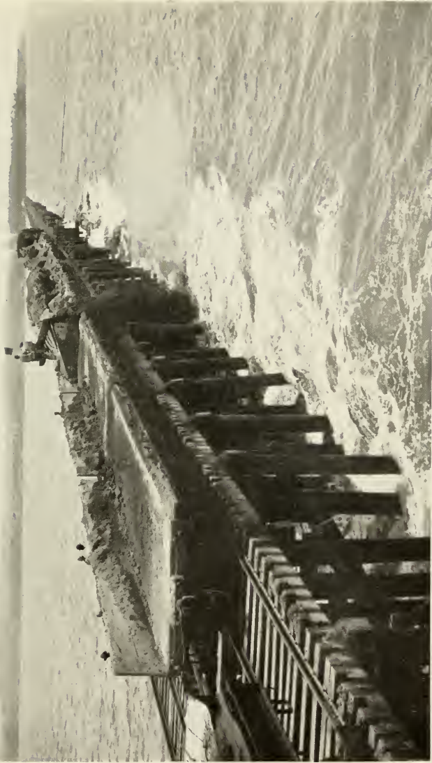
BUILDING THE BREAKWATER TO PROTECT THE ATLANTIC ENTRANCE TO THE CANAL, JULY 21, 1911.
